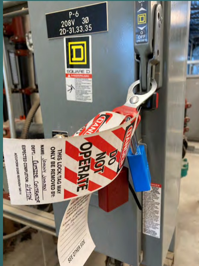
Step 2 – if contractor working on equipment, place lock and tag to scissor
